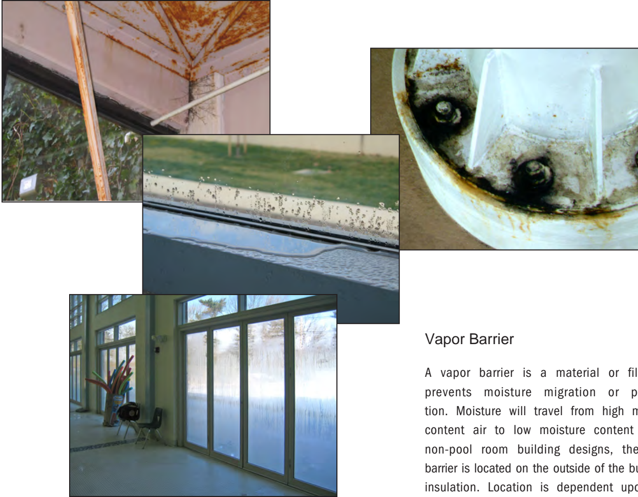
Figure 3. Examples of condensation and poor air distribution
