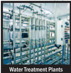
Water Treatment Plants
