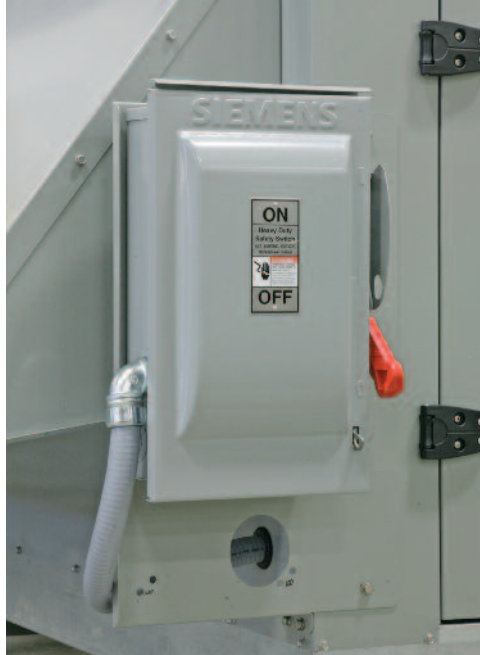
Figure 5 - Disconnect Switch Installed on Aura™ Series Unit
